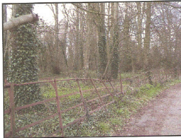
Fig 13 Damaged boundary fencing
